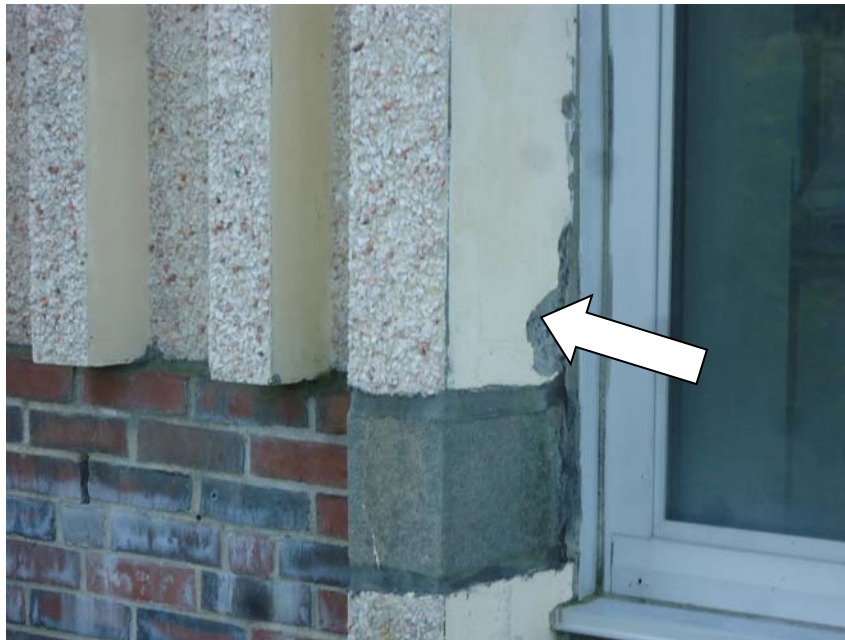
10. Precast panel spall along the aluminum window jamb. It appears that small portions of precast panel have been replaced
