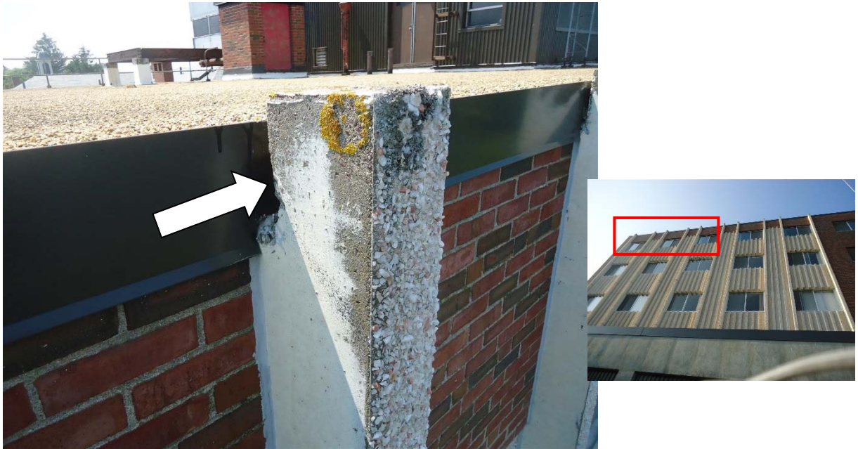
9. Precast panel ribs extend above the roofline on the east side of the north elevation. The existing configuration of the roof fascia onto the precast panel may result in accumulation of water in the gap between the panel and sheet metal.
